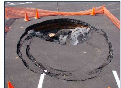
Sinkhole in parking lot overlying stormwater infiltration basin
